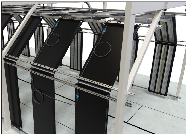
LEINS3 shown with DALI cabling
